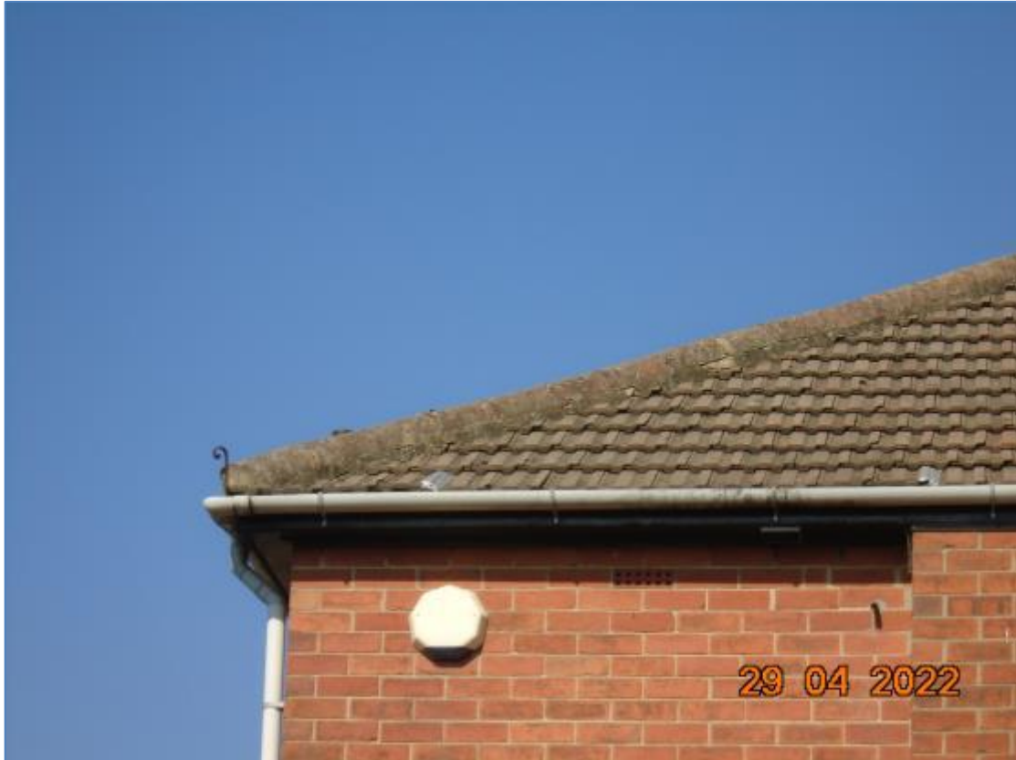
Photograph 3 – Shallow gaps under the rear elevation roof tiles.
