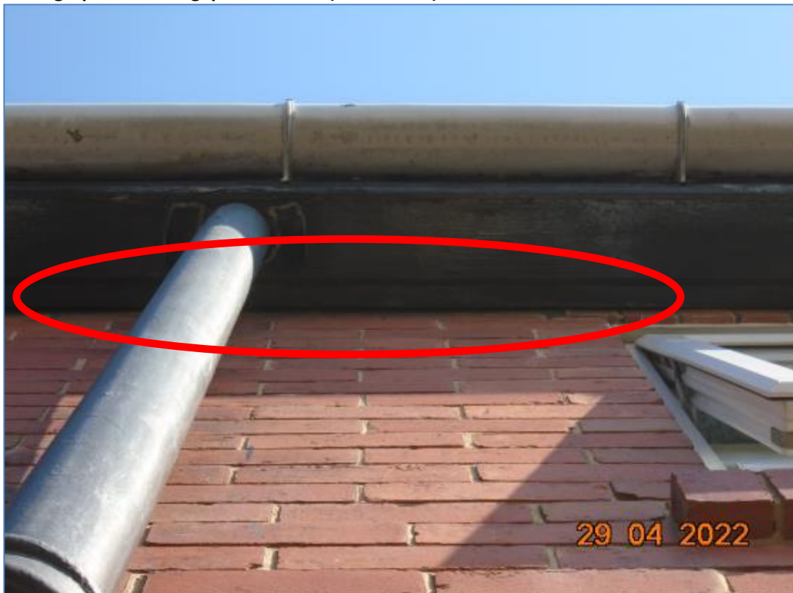
Photograph 4 – Soffit gap on the side (south-west) elevation.
